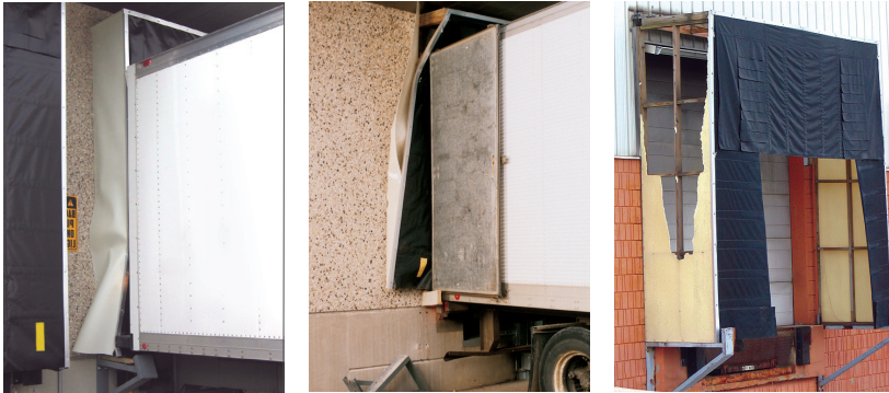
Just one trailer impact can severely damage or even destroy ordinary rigid-frame dock shelters.
