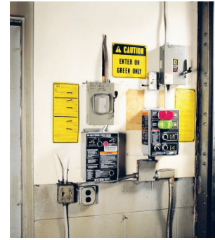
Multiple controls at each dock position can be complicated and potentially dangerous
